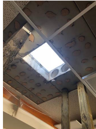
Siebert roof penetration
