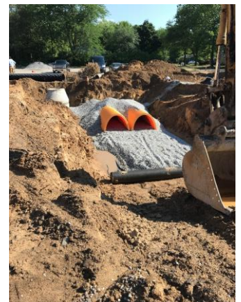
Underground retention system installed at Chestnut Hill
