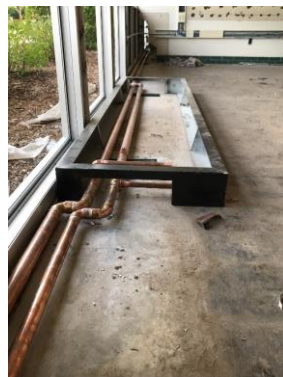
Unit ventilator piping set at Chestnut Hill
