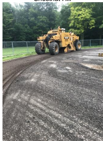
Siebert parking lot pulverized
